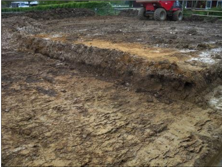
Plate 5: Plumpton Sandschool: Site showing stratigraphy of second ground reduction strip; looking northeast
