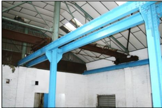
Plate 11: Building A Hoist
