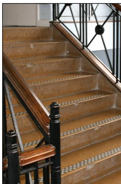
Plate 12: Chips in Polished Concrete finish on Stair Treads
