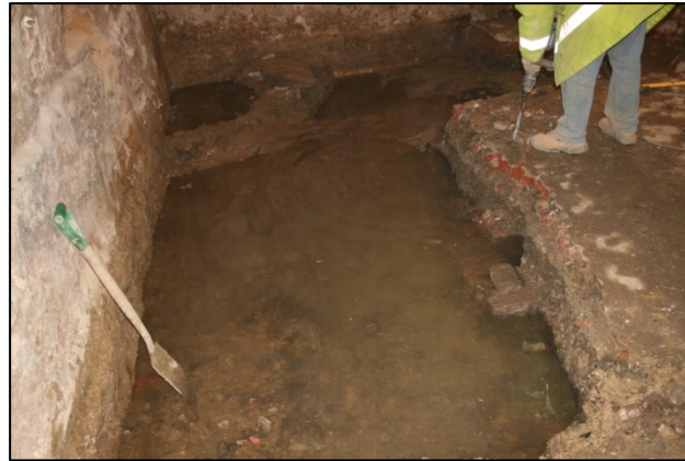
Plate 3: Ingress of water in cellar
