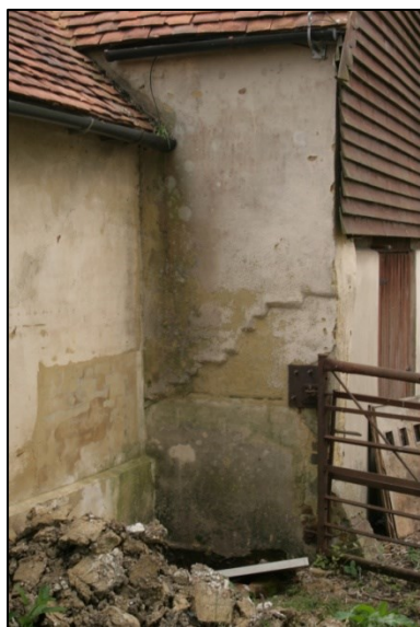
Plate 6: Possible Repair Western Side of North Wall
