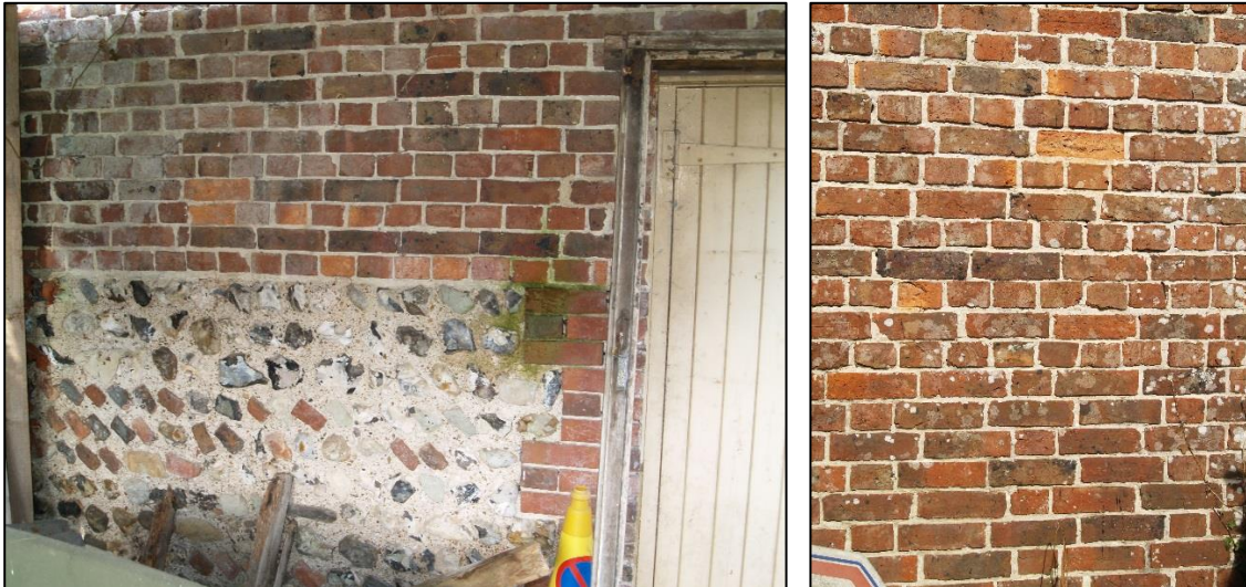
Plate 9 – The northern elevation of G2, showing low level flint wall with English bond brick work above at the western end, and the wall to the east of the central doorway note the lower Flemish Garden Wall (Sussex) bond at the base and the change to English bond above.
