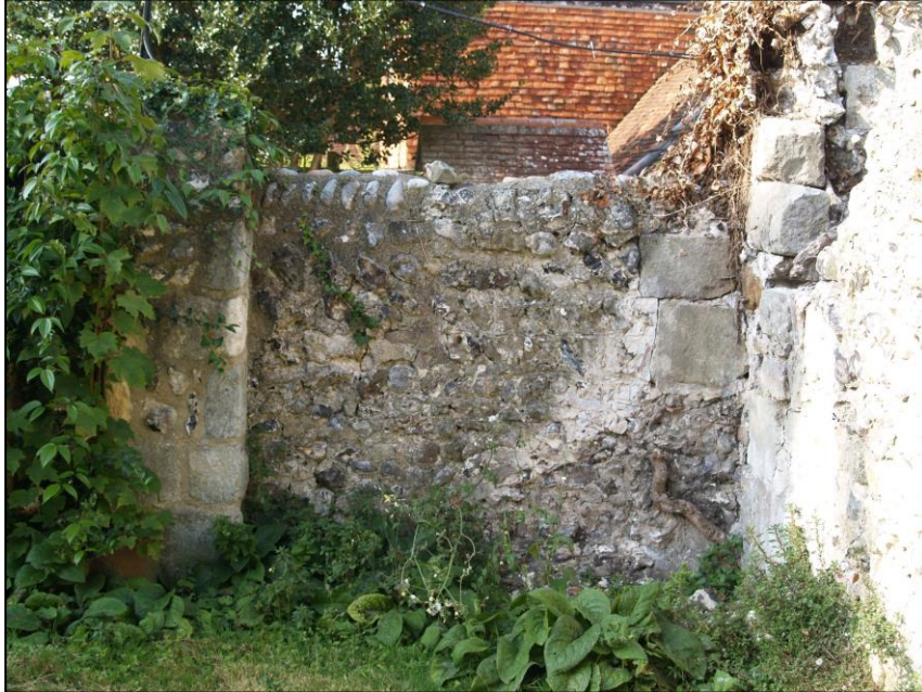
Fig. 4a – The blocked gateway in the western boundary wall immediately adjacent to the southern elevation.
