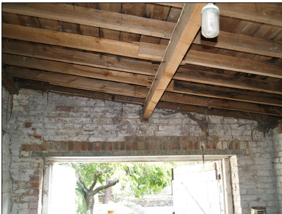
Plate 7 – The eastern internal elevation of G1 showing the Stretcher bond brick construction, modern door lintel and bracket holding the roof beam.
