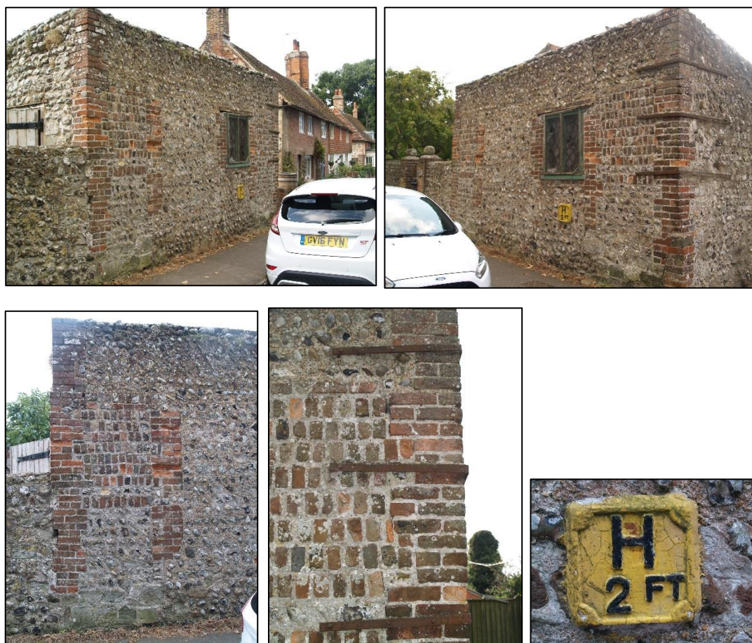
Plate 1 – The north elevation viewed from the east (top left) and west (top right). Note the long & short brickwork at each corner with the adjacent infill columns (detail bottom left) the NW corner metal strapping (bottom middle) and detail of the 'Hydrant' sign (bottom right).
