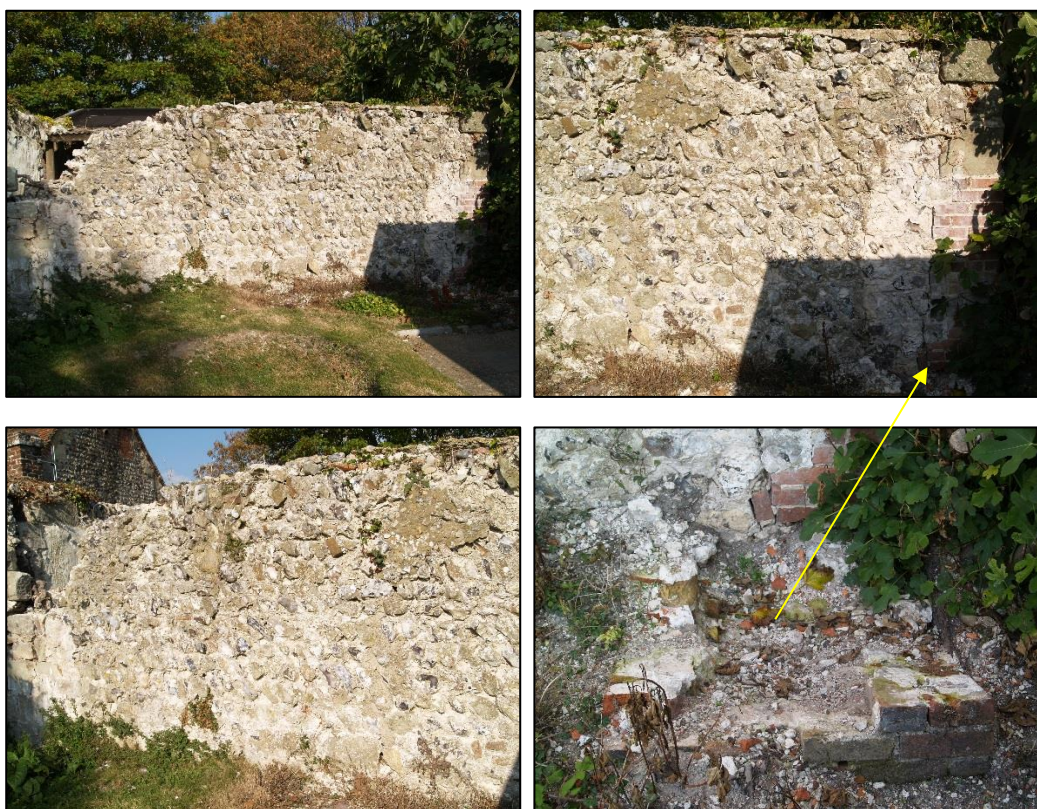
Plate 4 – The southern elevation, showing a general overview (top left), detail of the eastern end (top right), note the brick feature at the base and the mark on the wall directly behind. The western end (bottom left) and detail of the brick feature at the eastern end (bottom right).
