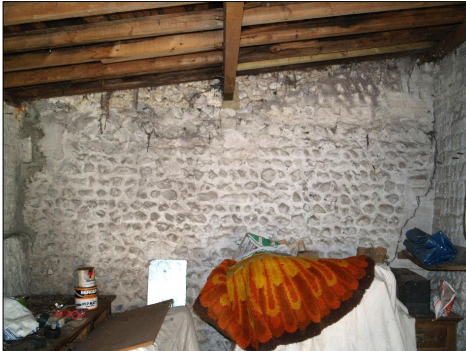
Plate 5 – The internal western elevation showing the coursed flint on the lower part of the wall with more randomly coursed flints above, the brick column in the NW corner and the modern roof timbers.
