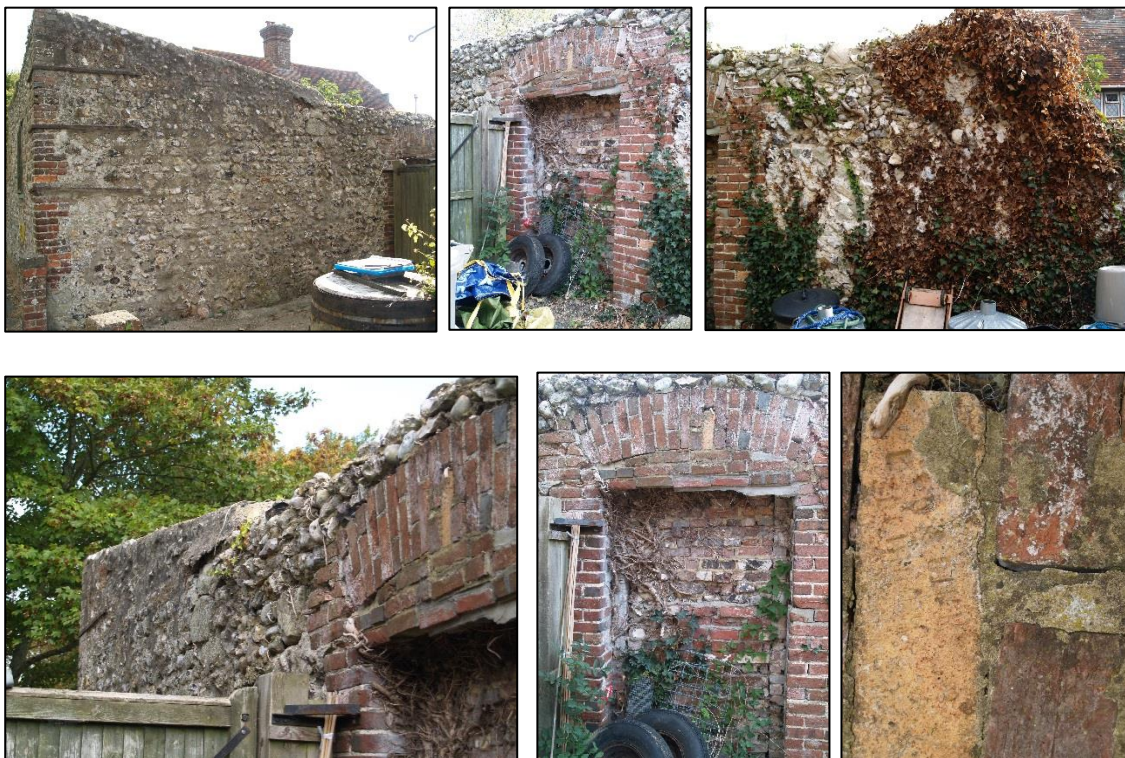
Plate. 2 – The Western Elevation viewed from No. 94, High Street, The NW corner showing the coursed flint construction with the added upper phase supporting the flat roof of G1 (top right). The infilled doorway with its brick supporting columns and arch (top centre) and the southern end of the elevation constructed in larger flints (top right). Detail of the ' Rubble ' flint work above the arch (bottom right), detail of the blocked doorway showing the brick jams (bottom centre) and detail of Marker mark on one of the arch bricks (bottom right).
