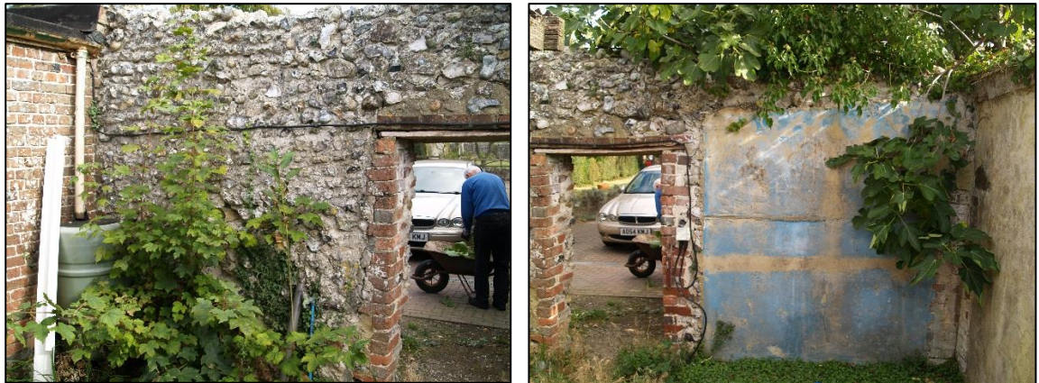
Plate 11 –East elevation of G2,north end (left) to south end (right), note the area of rendering on the south of the elevation which corresponds to similar on the west elevation, denoting where a lean-to formally stood.
