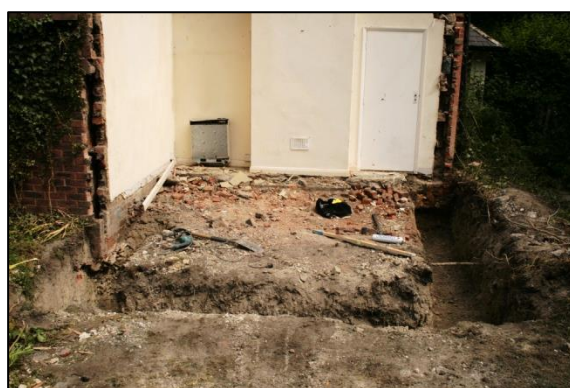
Plate 1: The Excavated Footing Trenches for the South-Eastern Extension taken from the South
