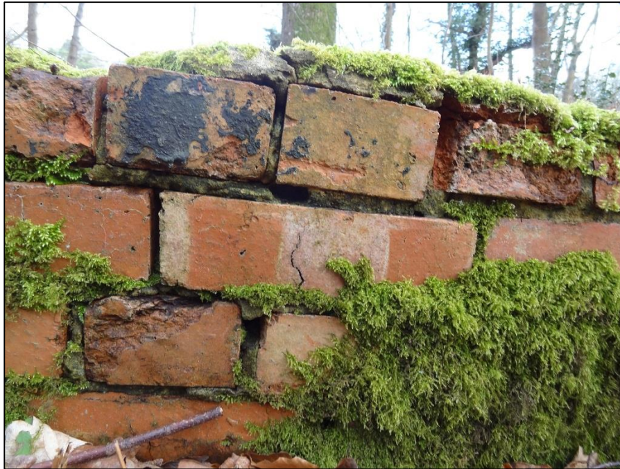
Plate 41 – Detail of the remaining wall of feature SP.067 showing the state of preservation.
