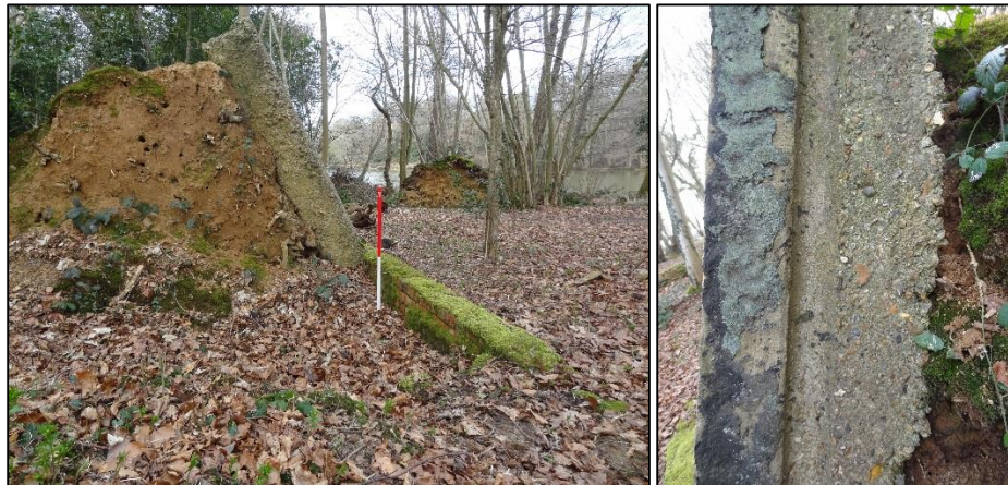
Closer view of the uprooted slab showing the thickness of concrete (above left) and a close up detail of the groove fabric of the concrete base (above right)
