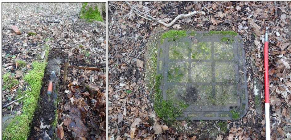
Water supply pipe in NE corner (above left) and drain cover adjacent from south wall (above right)
