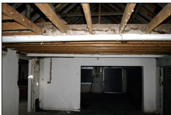
Plate 13: Exposed Joists in G2
