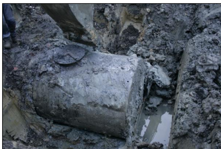
Plate 27: Petrol Tank in Trench 2
