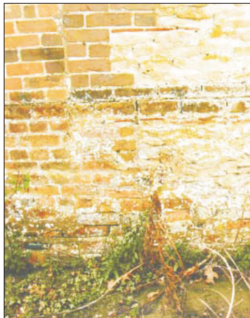
Plate 12: Quoin of phase one with water table. Later (18th century) build to left (west) south front.
