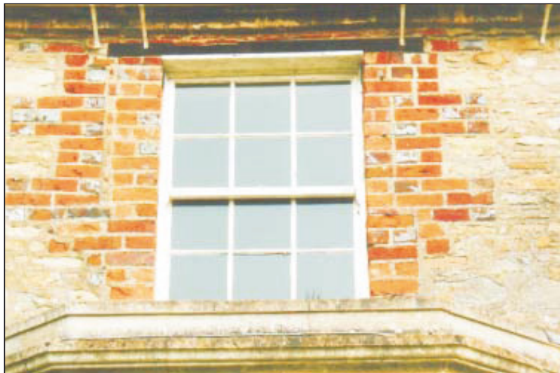
Plate 6: First floor window in south front of first phase building. Note the straight joints indicating that the window was formerly wider and shorter.
