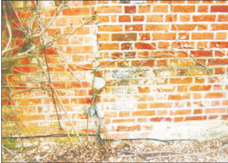
Plate 9: Detail of the south front showing the second phase (brick with stone footings) and the junction with western extension.
