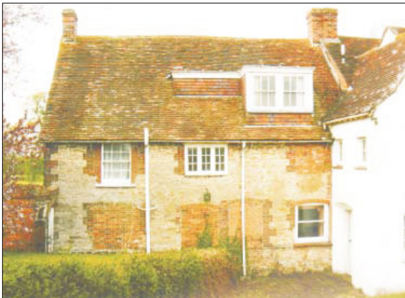
Plate 10: Rear, north elevation at east end. Note the blocked windows and doorways, also the early window in the centre of the first floor.
