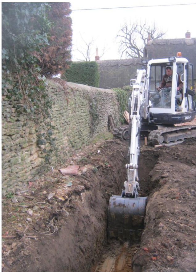
Figure 2. The machine excavation of one of the new footing trenches along the eastern side of the Site.
