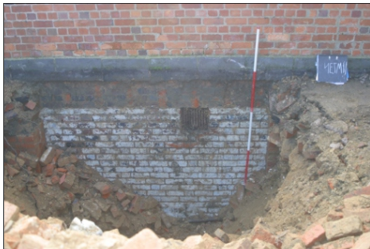
Figure 4. Excavation of cellar showing east wall of cellar, ventilation grill and shadows of floor joists.
