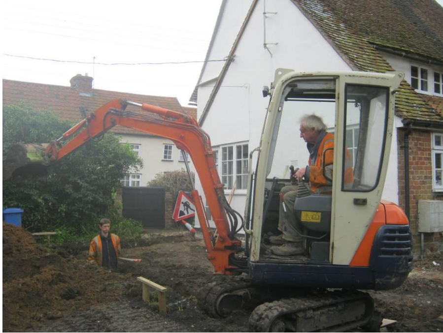
Figure 2. Machining the footings trench on Site on the 15 th May 2012, looking south-west towards the existing building and Bolton Street.
