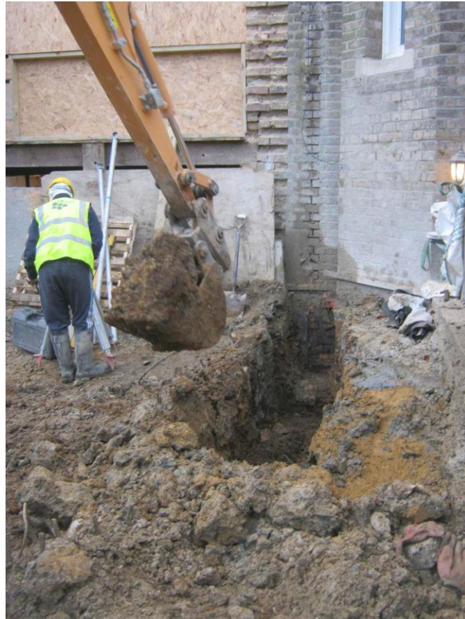
Figure 2. The initial phases of excavation of an extension to the current cellar at the rear of the existing building
