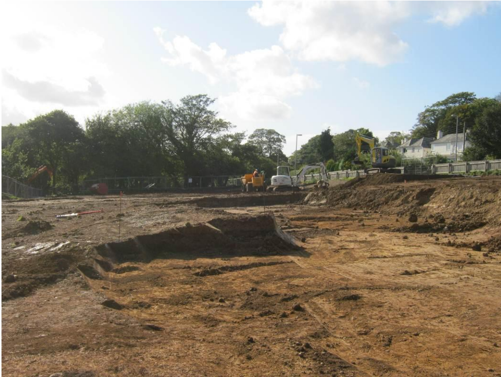
Plate 1. Machining and groundwork in Area 2 looking north-west, showing the increasing depth of colluvium and made ground towards Tinney Drive.
