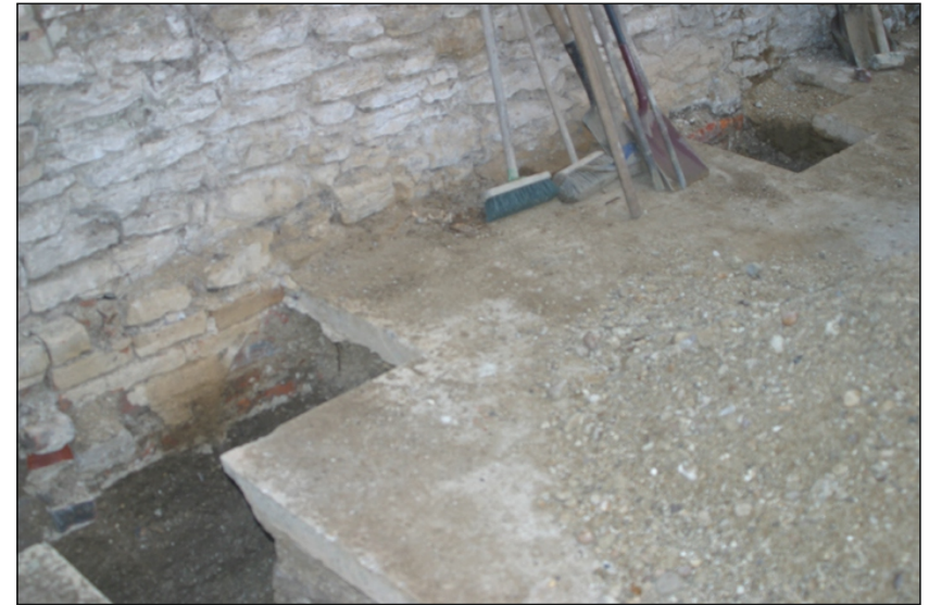
Figure 4. Photograph of footings trench showing walls 2 (located on extreme left of photo) & 3 (within footings trench).
