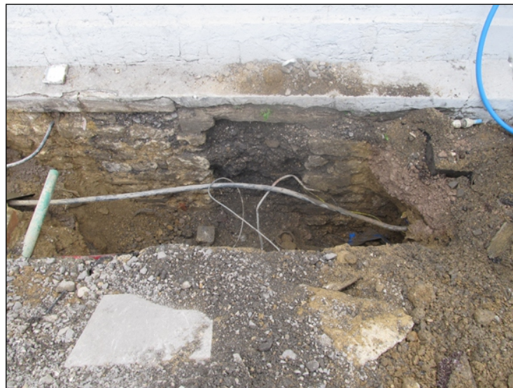
Figure 5. Photograph to right showing line of wall-footings 105 of toll booth and location of access observed during watching brief.
