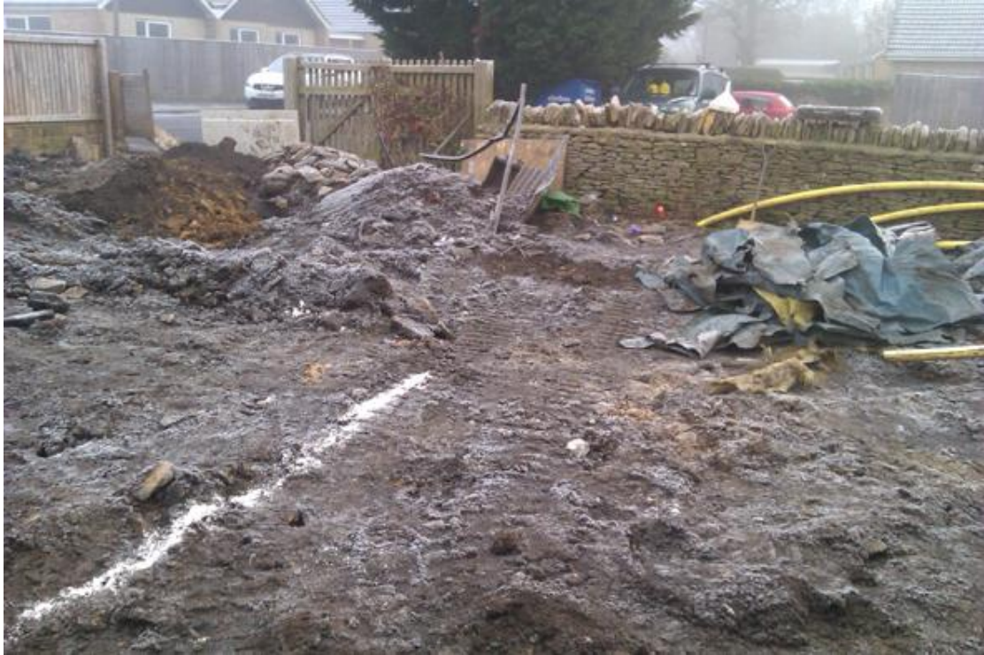
Figure 2. Investigation area, showing dumped building materials at rear next to gate.
