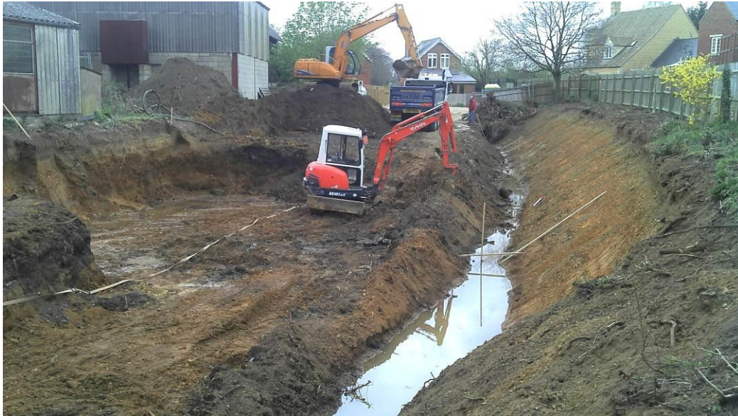
Figure 2. Photograph of the Site on the 3 rd April 2012 looking north, showing the large quantity of material removed without monitoring at the southern extent of the development area, and the large open drainage ditch along the eastern boundary.
