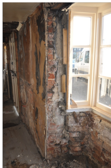
Plate 22. Butt joint in bay windows, Structure A
