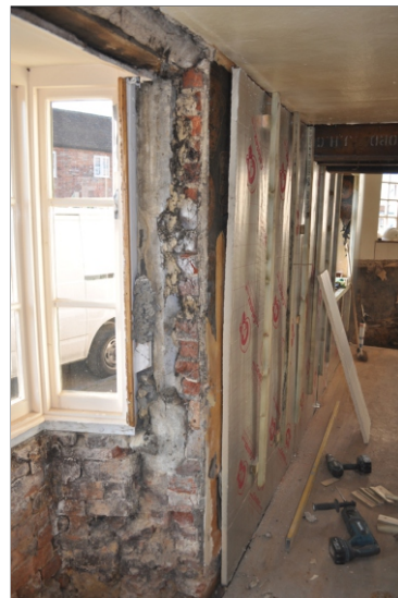
Plate 21. Butt joint in bay windows, Structure A
