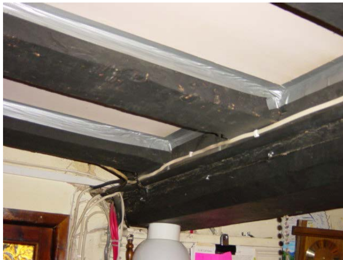
Plate 8: The continuation of the early spine-beam into the office, with ceiling joists in situ
