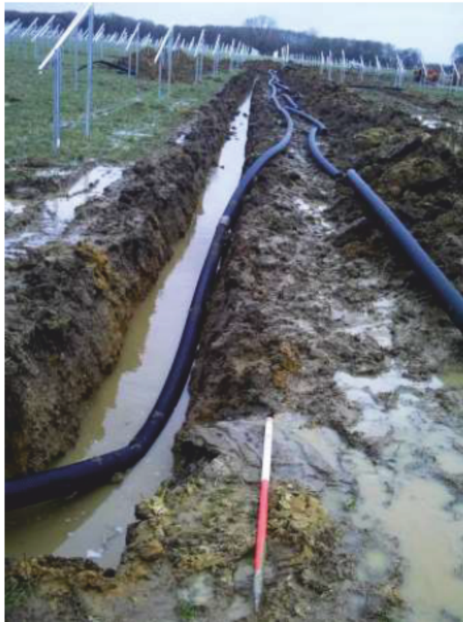
Figure 3. Cable runs; looking west.
