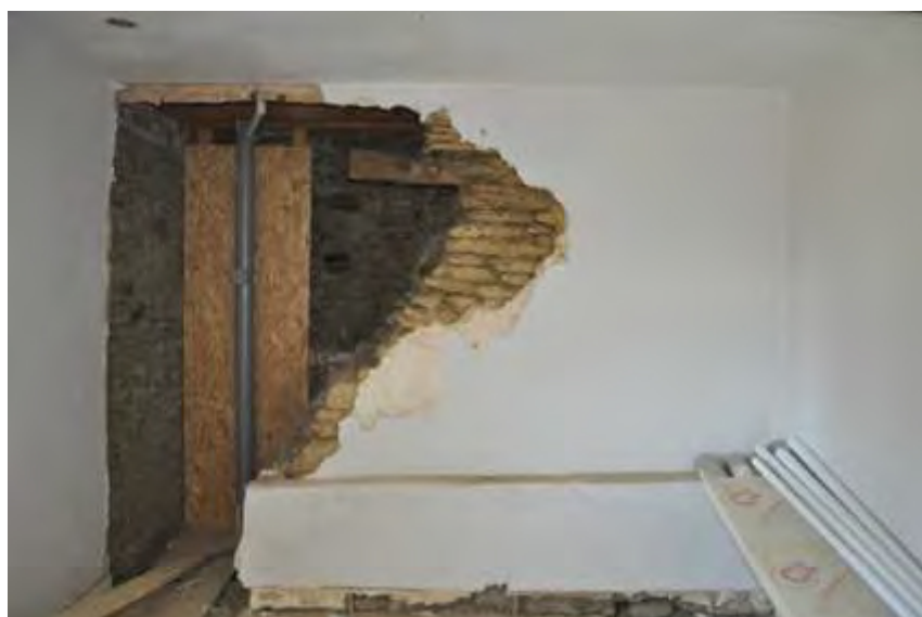
Plate 14: Chimney breast edge in bedroom 2
