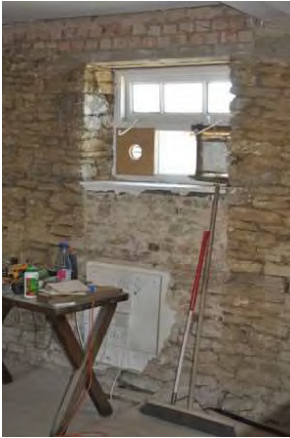
Plate 17: Partially blocked window in office.
