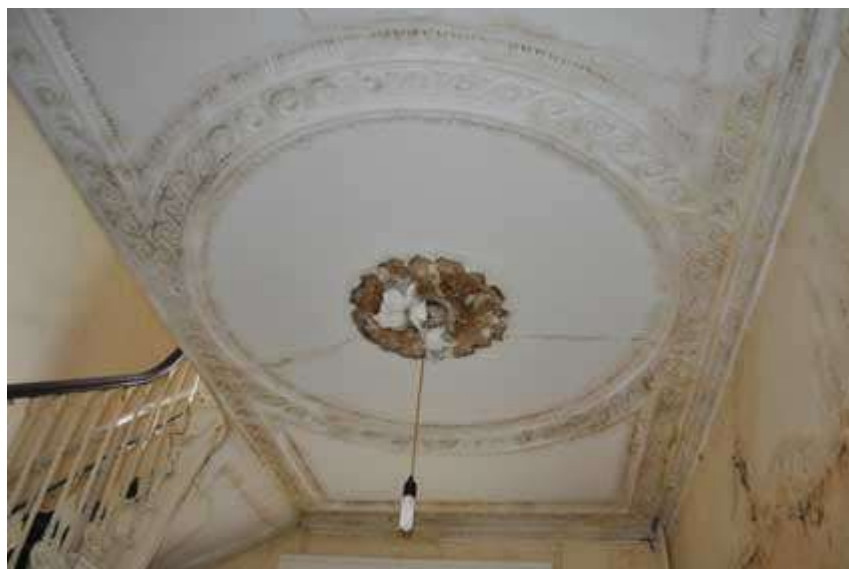
Plate 11a Damaged hall ceiling
