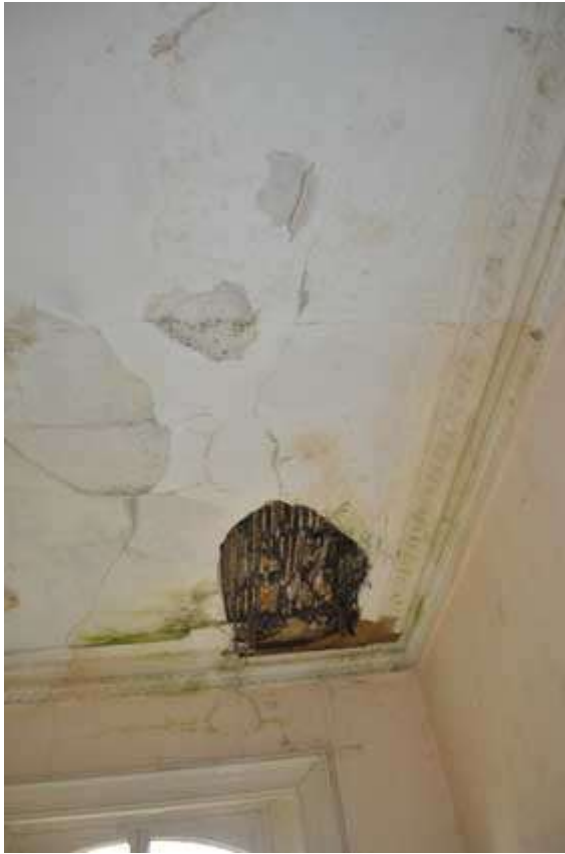
Plate 21a Landing showing damaged plaster
