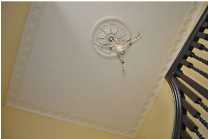
Plate 16: Ceiling above stairwell
