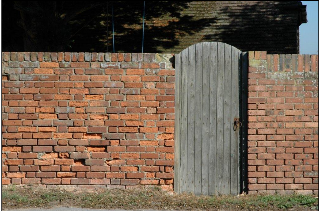
Fig 17. The junction at an original gateway between the Speen Manor garden wall and the recent replacement of a section of it where the land has been sold off.
