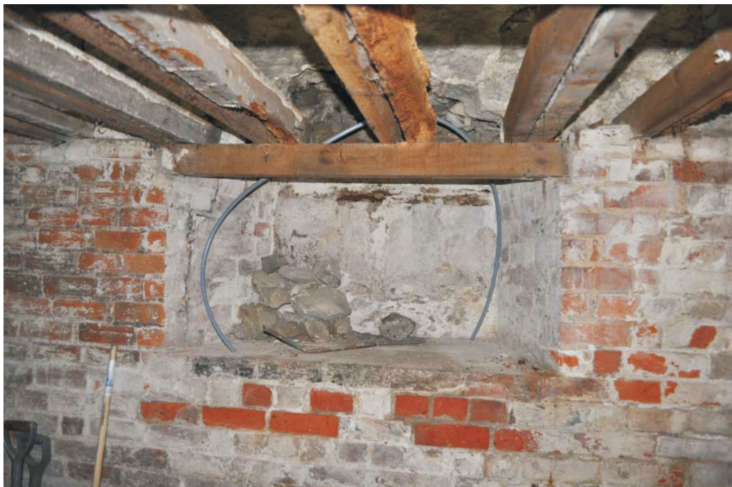
Plate 10: Blocked up window in the cellar
