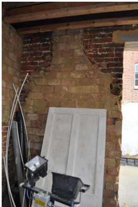
Plate 9 RE5 blocked flue in wall
