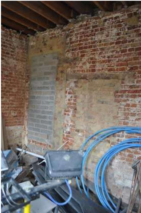
Plate 8 RE5 blocked doors
