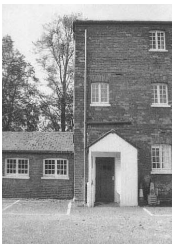
Plate 35: Inserted window at first floor level
