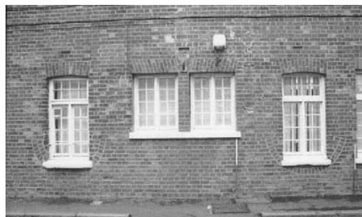
Plate 34: Inserted modern window in west elevation of West Wing also shows inserted (or extended) Type 4 windows
