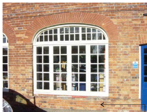
Plate 16: The Inserted Type 3 window in the West Spoke showing English bond in the in-fill
