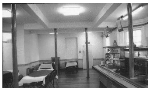
Plate 12: Cast Iron Columns in Central Hub (shows the beams they are supporting)
