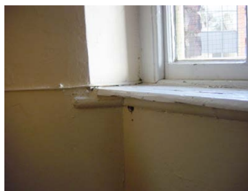
Plate 14: The 'swept round' original windowsill under the later replacement
