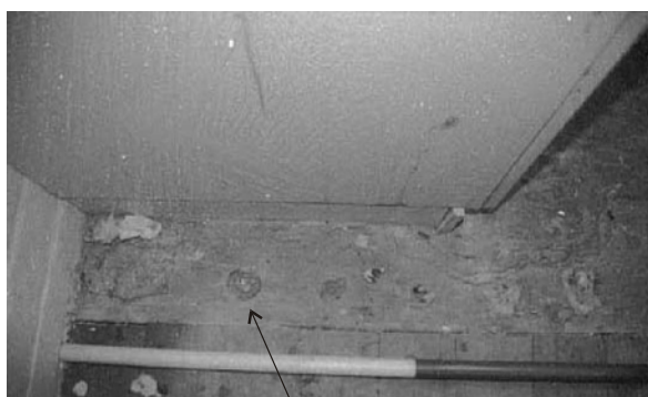
Plate 19: The slab of original stair landing showing locations of removed banisters (arrow) and boarded over access
