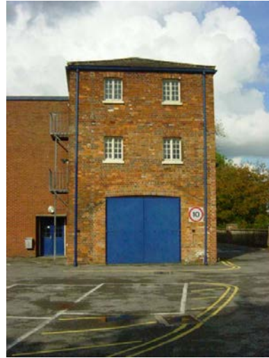
Plate 21: Inserted door and scar indicating location of original southern extension to the East Wing
