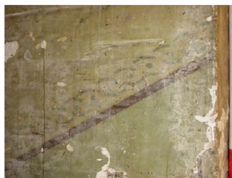
Plate 20: The remains of paint finish at the top of removed original stairway in the East Wing
