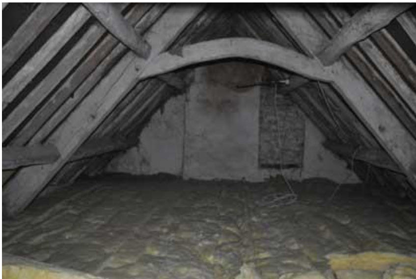
Plate 10 Bowed cross beam (A5)
