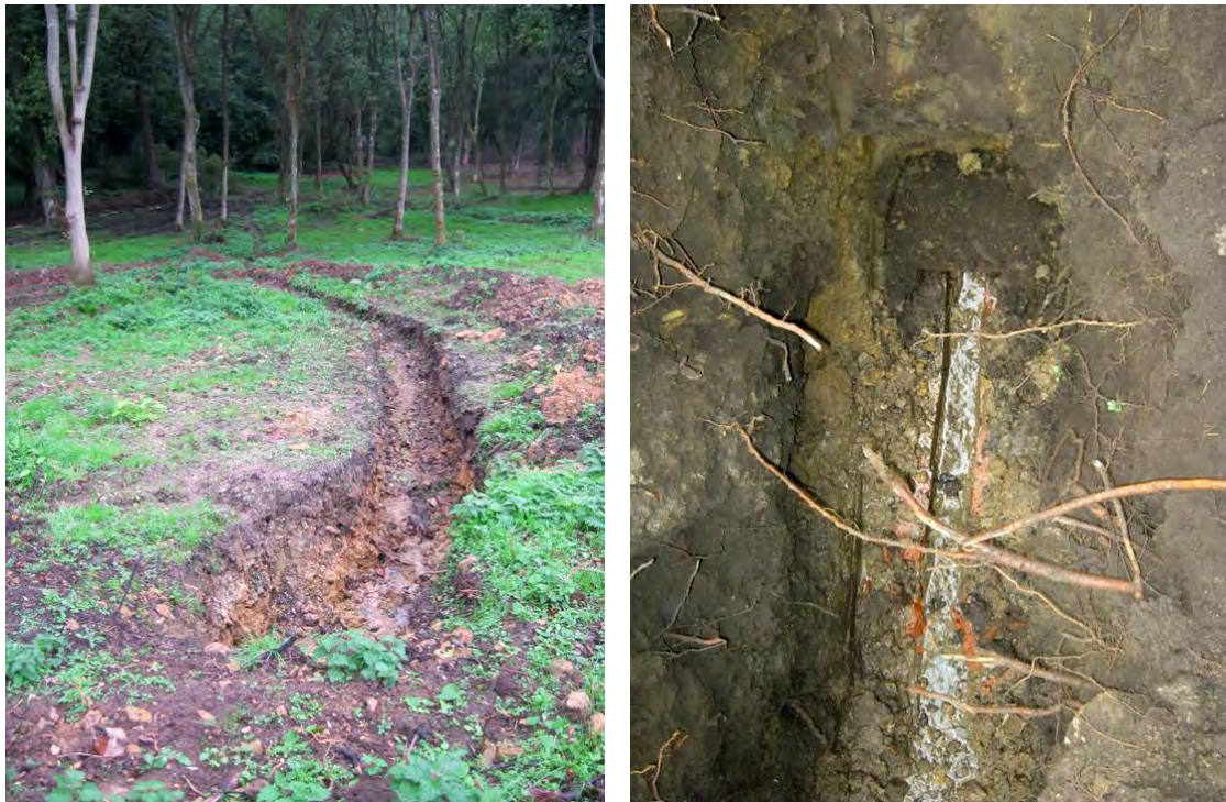
Plates 2 & 3. Drains in the “wilderness” area
