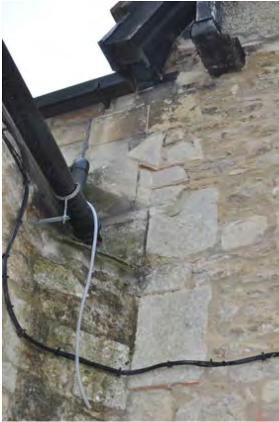
Plate 4: Remains of diagonal buttress on north façade
