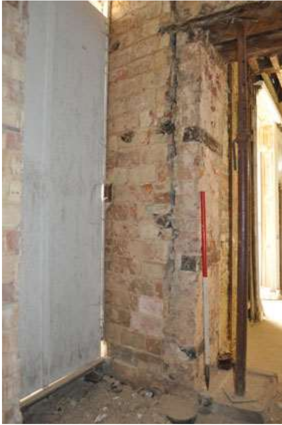
Plate 8: G15 butt joint in S wall
