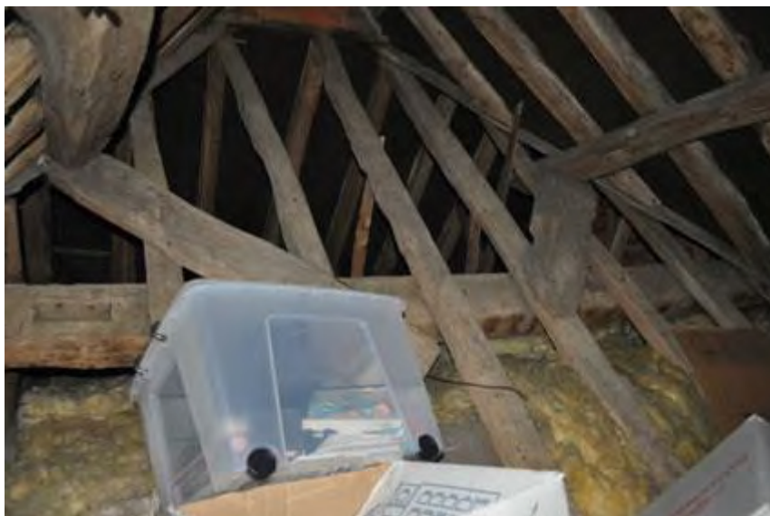
Plate 25: Timber frame of northeast range being built onto by later roof structure
