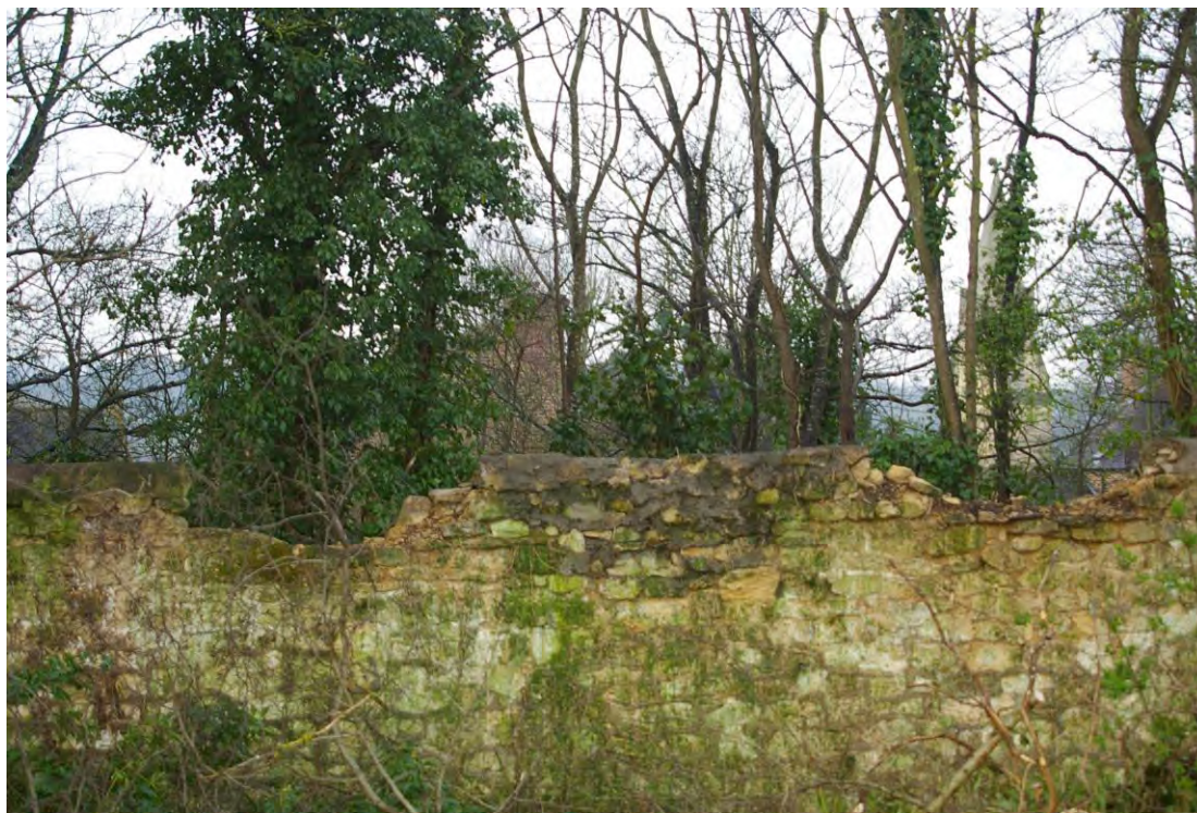
Plate 7. Damage to upper section of wall 100
