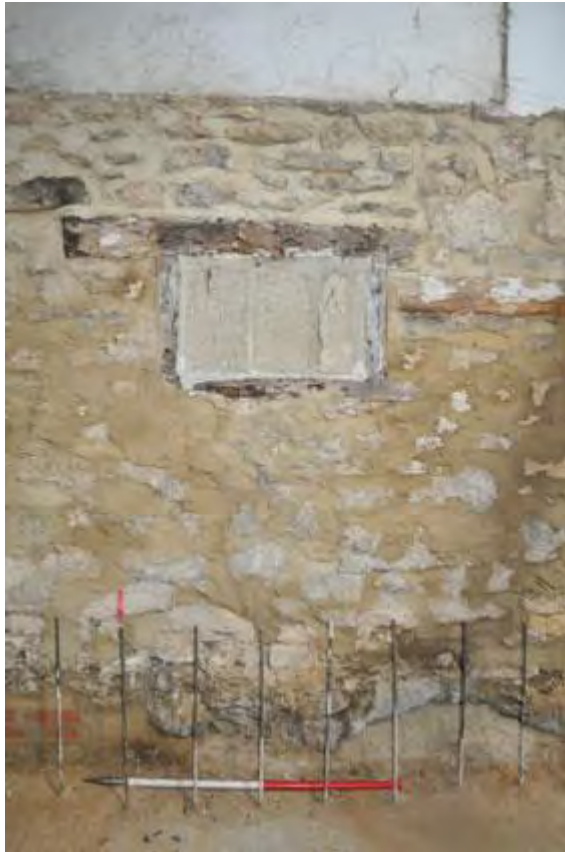
Plate 12: Part of wall 18 (with collapsed foundation)
