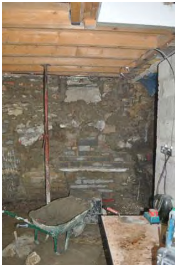
Plate 14: Part of wall 18 (after collapse) with wall 48/76 removed (on right)
