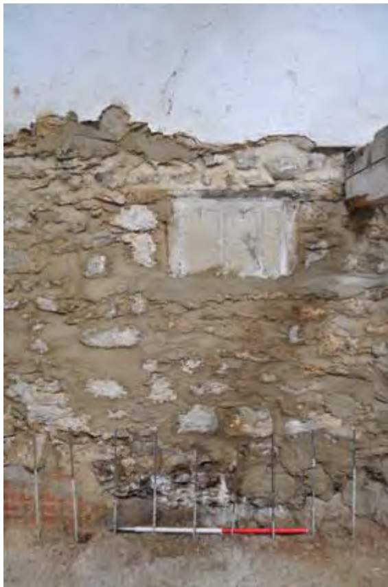
Plate 13: Part of wall 18 (with collapsed foundation)
