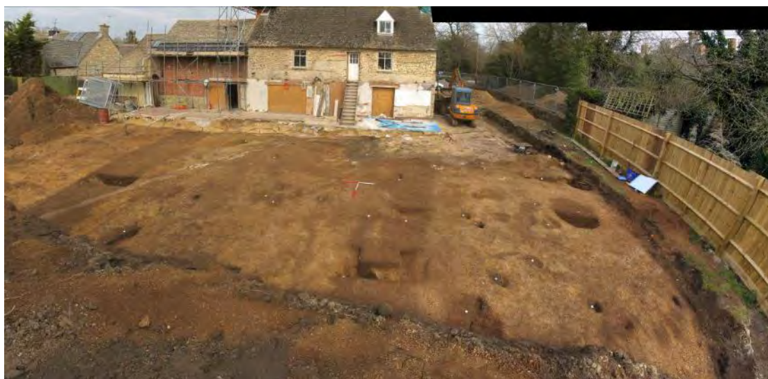
Plate 1: General view of the backyard area (before further extension to the SW corner)
