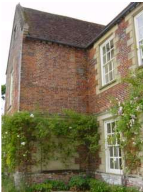
Plate 1: Blocked windows both of which are proposed for re-installment
