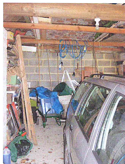
Plate 6: The 1980s breeze-block reinforcement of the southern gable wall
