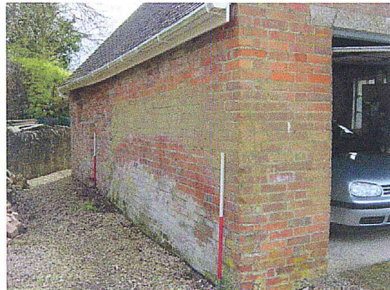
Plate 2: The distorted east wall
