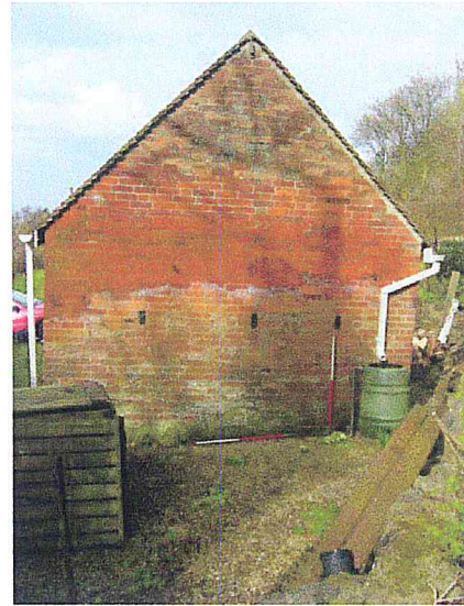
Plate 1: Southern gable showing iron-work associated with pigsties
