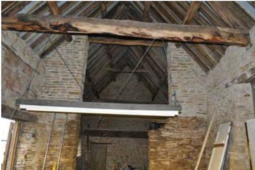
Plate 15: Blocked window in the west wall
