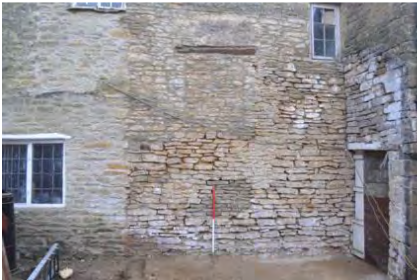
Plate 19: Blocked window near stairwell
