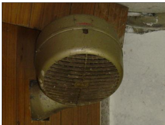
Plate 12: Wall mounted fan heater
