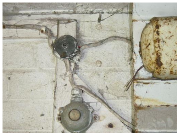
Plate 11: Detail of switches, junction box and cable
