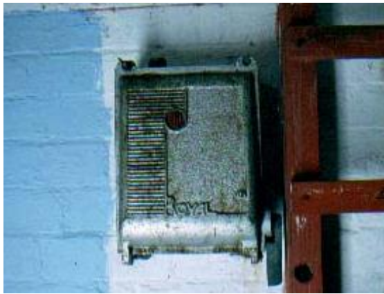
Plate 10a: External view of fuse box
