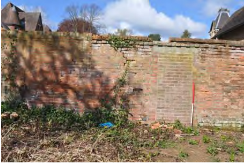
Plate 14: Blocked entrance and joint in Wall 1 (view to west)
