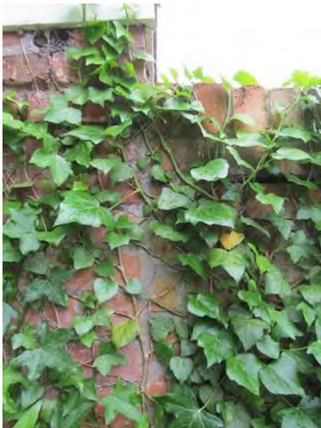
Plate 7: Joint in Wall 1 at north edge of garage
