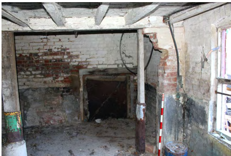
Plate 17: Southern building, access point to room G2 in western wall of room G1.
