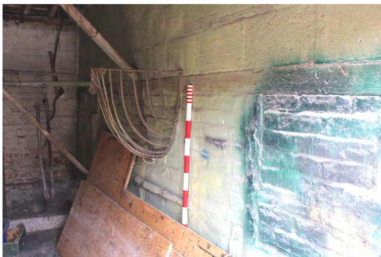
Plate 8: Northern building, original partition with later concrete block extension in room G2.
