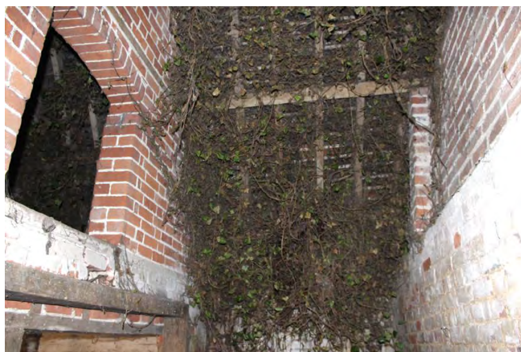
Plate 23: Southern building, access between rooms G1 and F1 at western end of room G1.
