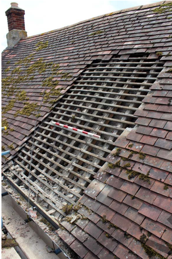
Plate **: Area stripped prior to removal of roof fabric and dormer window insertion
