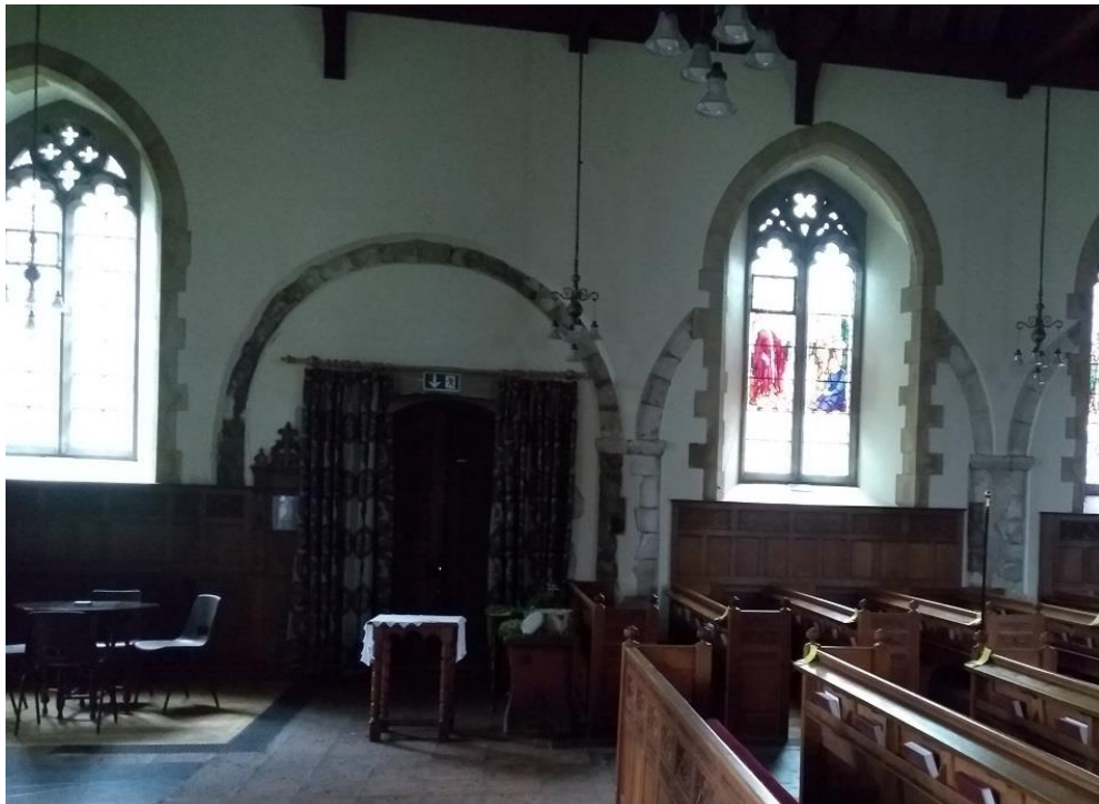
Plate 2. Interior view of St. Mary's Church, Wargrave. An archway associated with an earlier architectural layout of the church, potentially corresponding to the flint masonry uncovered perpendicular to the archway on the external side of the wall. View facing north.
