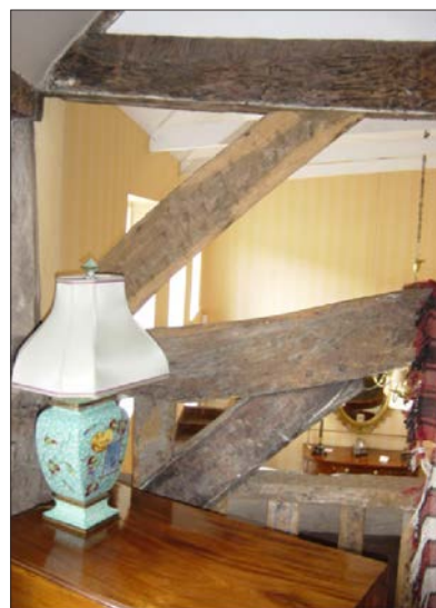
Plate 12: The remains of the timber framed west end wall of the cottage
