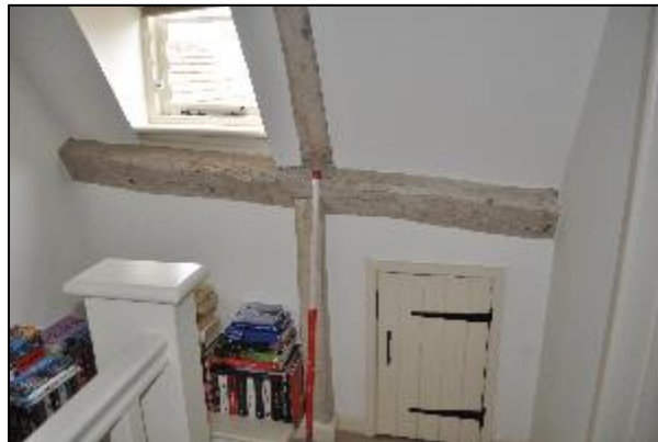
Plate 25 The single casement window and the exposed beams in the northern wall of S1.
