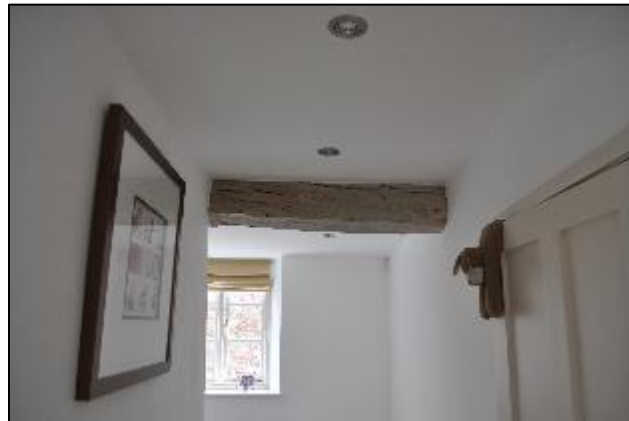
Plate 27: The chamfered beam in the ceiling of F5, which connects to the beam seen in F5 (Plate 26 above).
