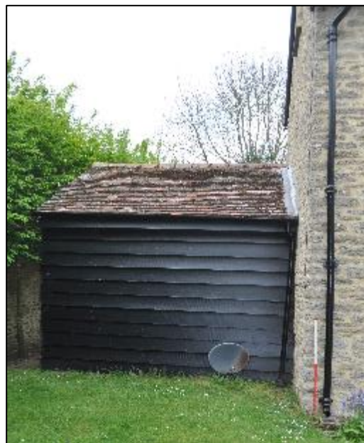
Plate 6: Area 2 of Southern Elevation comprising the modern kitchen wing attached to the Main House (Area 1)
