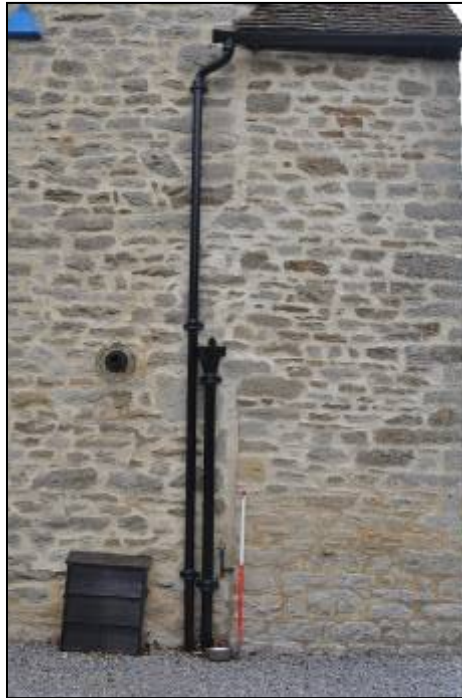
Plate 8 The butt joint is visible to the right of the drain pipe in E3: Eastern Elevation
