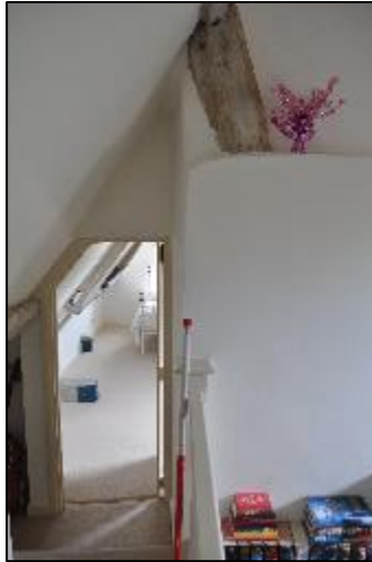
Plate 33: The Western wall of S1 looking towards the doorway into S2. An exposed brace beam can be seen above the chimney wall.
