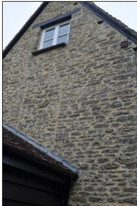
Plate 11: The Second floor window of E4: The Western Elevation showing the two vertical joint lines where windows were likely removed.
