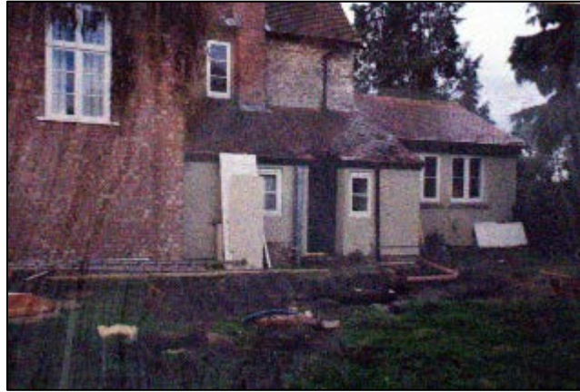
Plate 16 The Northern Extension c1999 prior to the demolition of a previous lean-to and boiler and the addition of Face Wing 3. Note that Face Wing 2 wall has yet to be rendered in cement at this point but the kitchen extension G3 has been built (Image Courtesy of Mr Minoli).
