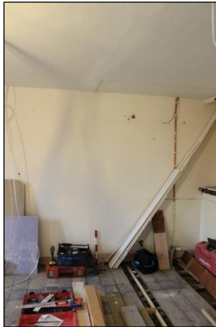
Plate 9: The Location of the Doorway prior to removal in Room 1:3. Note the service pipes under the floorboards. Just visible the dark line of the earlier removed wall
