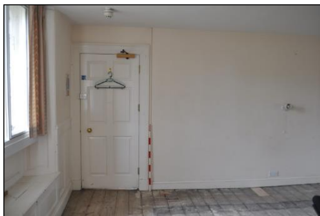
Plate 7: The main door, and just visible on the floorboards the remains of a possible earlier wall
