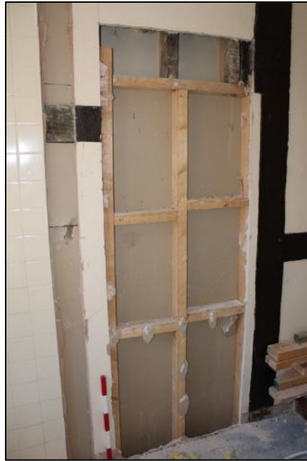
Plate 11: The Exposed beams below the plasterboard
