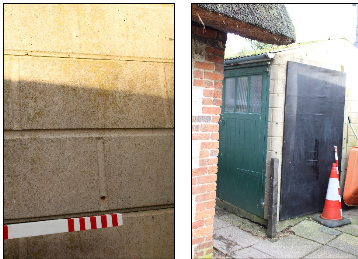
Plate 12: (Left) The poured and moulded concrete walls shaped to form bricks and (Right) the curved moulded corners
