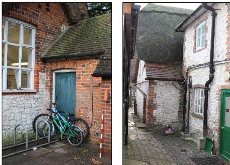
Plate 3: The Rear Elevation featuring: (Left) the northern classroom butted by the cloakroom extension. (Right) the central door of the rear elevation Main Schoolhouse and the southern classroom.
