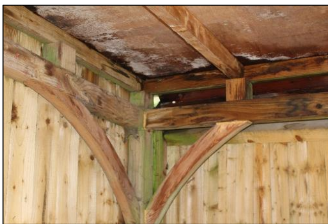
Plate 10: Interior of the corner of the bike store roof with the curved braces
