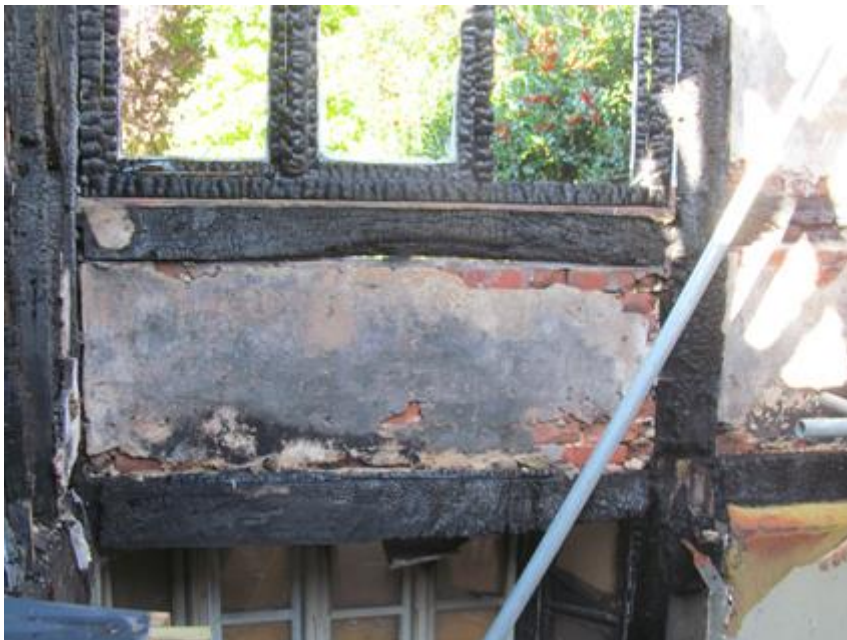
Plate 57: F3 west wall
